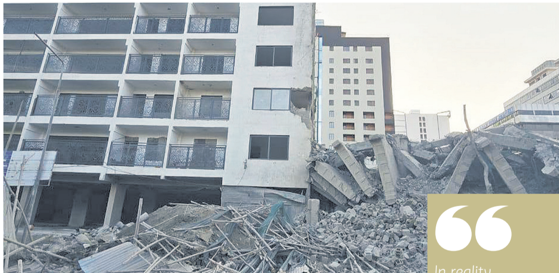
Part of the building that collapsed in South C, early this year. [Courtesy]
